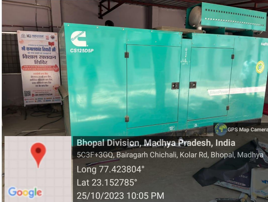
GENERATOR FOR BATTERY BACKUP
